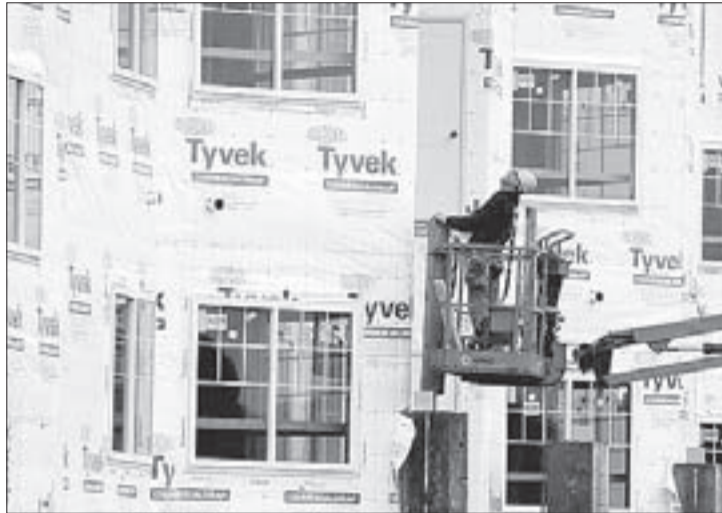
A construction worker works at a new home under construction in Chicago.
